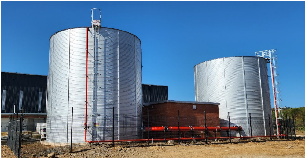
Photo above – Fire suppression tank system
